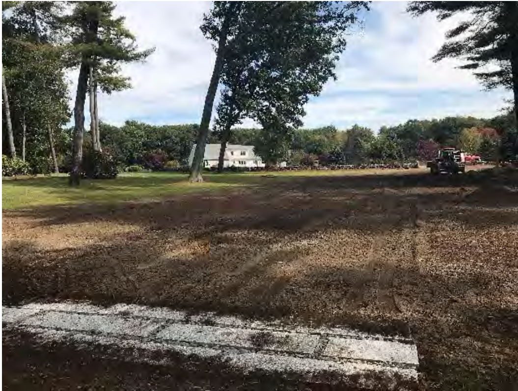
Fig 5: Spreading loam on the lawn above the slope at Gundalow Landing/east side of the bay. Viewing northeast. (09-28-20)
