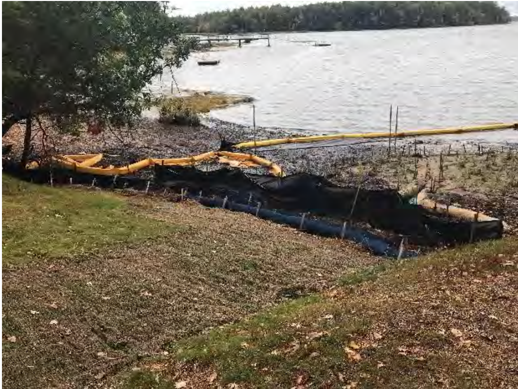
Fig 9: Toe of the slope below the manhole at Gundalow Landing/east side of the bay. Viewing south. (09-30-20)
