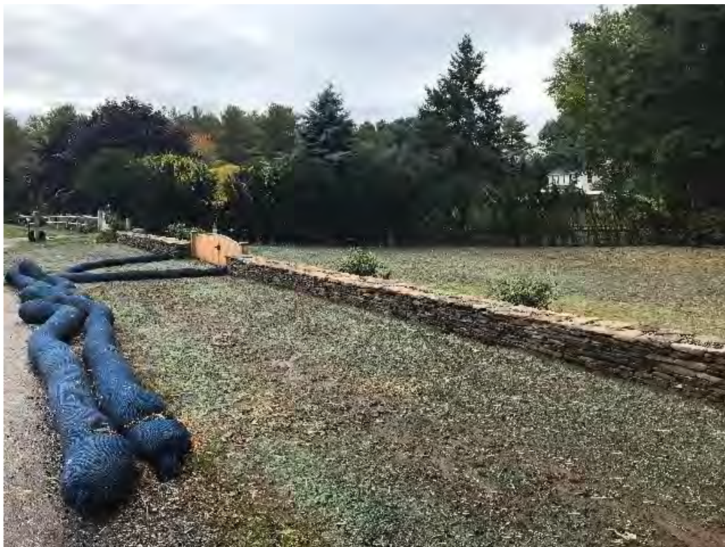
Fig 6: Loam and hydroseed spread on the lawn at Gundalow Lading/east side of the bay. Viewing southeast. (09-30-20)
