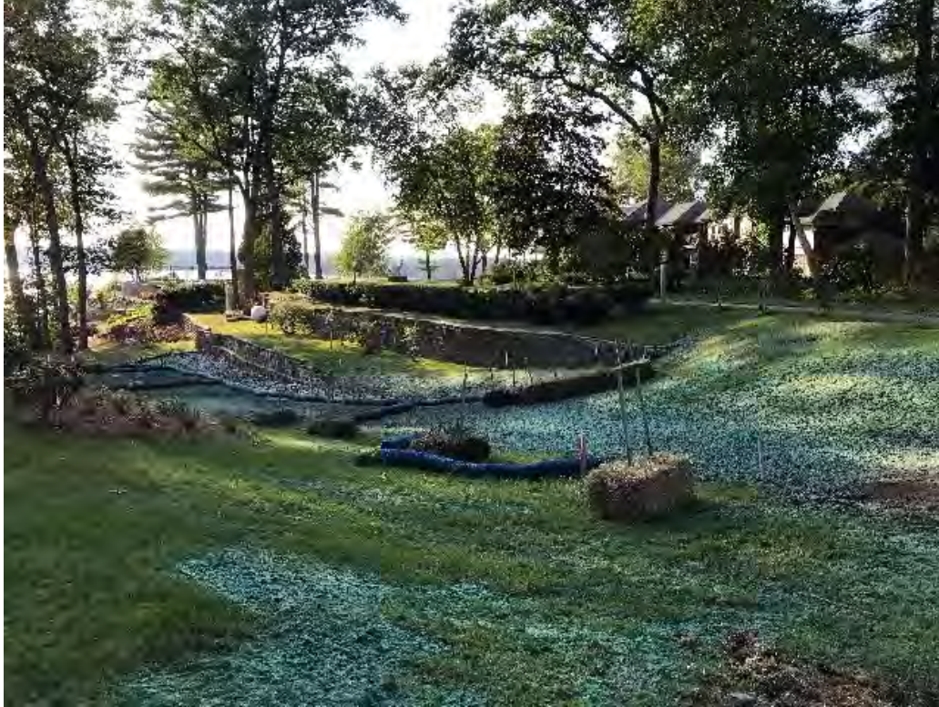
Fig 3: Hydroseeding the slope above the manhole at Gundalow Landing/east side of the bay. Viewing west. (09-25-20)
