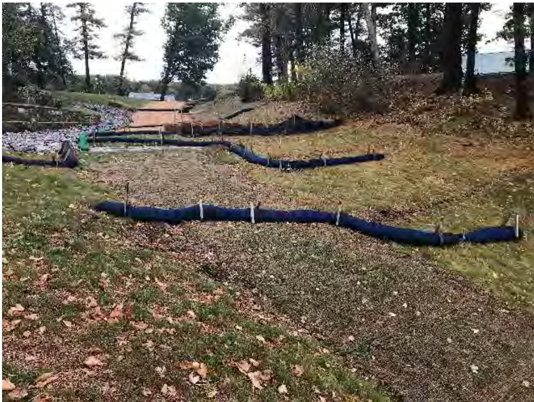
Fig 8: Slope below the manhole at Gundalow Landing/east side of the bay. Viewing east. (09-30-20)
