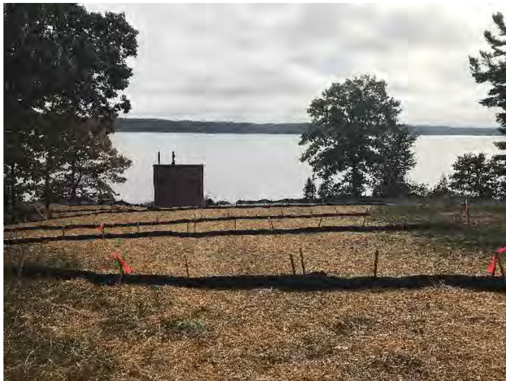
Fig 4: Straw and silt socks installed on the slope at the Eversource property/west side of the bay. Viewing east. (09-28-20)
