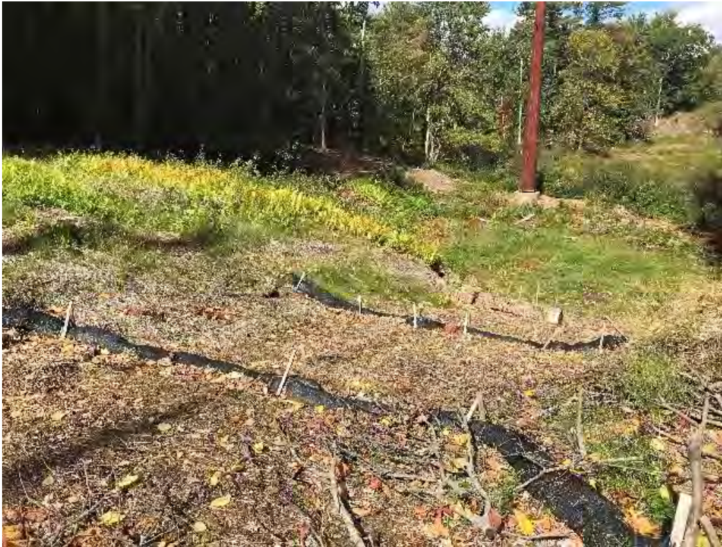
Fig 15: Swale between Strs. 28 and 29 is revegetating. Viewing northwest. (09-30-20)
