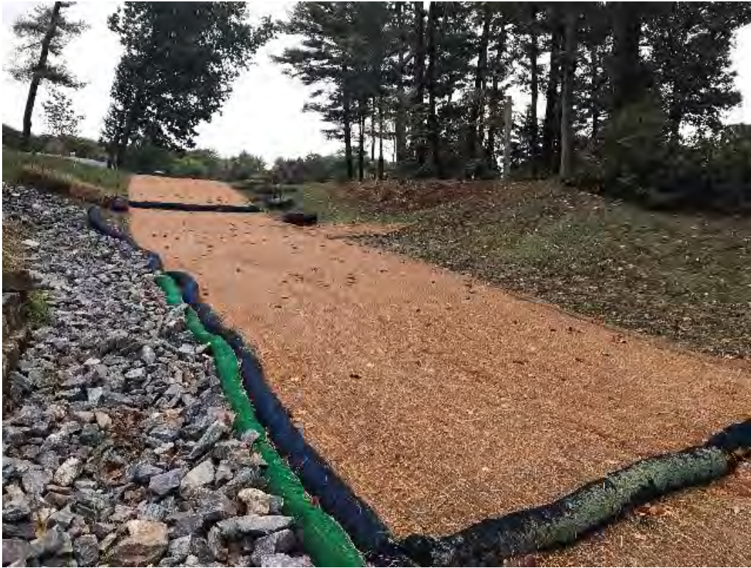
Fig 7: Jute matting securing the slope above the manhole at Gundalow Landing/east side of the bay. Viewing east. (09-30-20)
