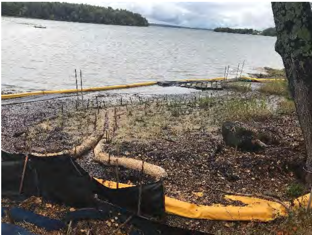
Fig 10: Salt marsh restoration at Gundalow Landing/east side of the bay. Viewing southwest. (09-30-20)
